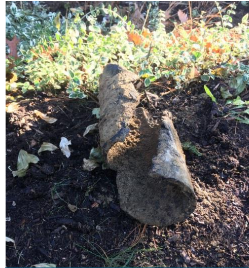
Failed piece of 4-inch Orangeburg pipe removed from septic system on Walker Lane. (Photo: T. Achituv)
