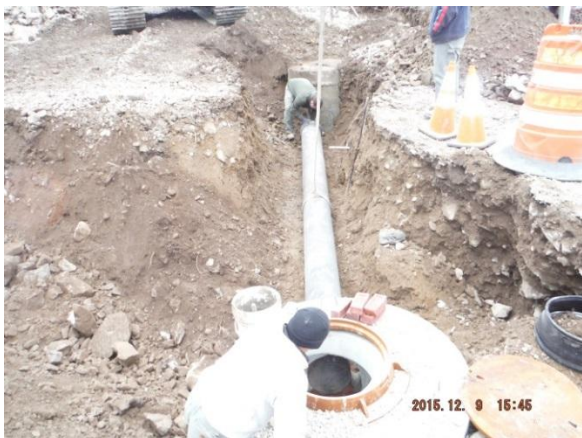
DCB 1 & DCB 2 connected to WQU 12/9/15
