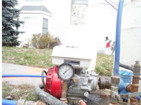
Water main pressure test fails due to minor leak 12/9/15
