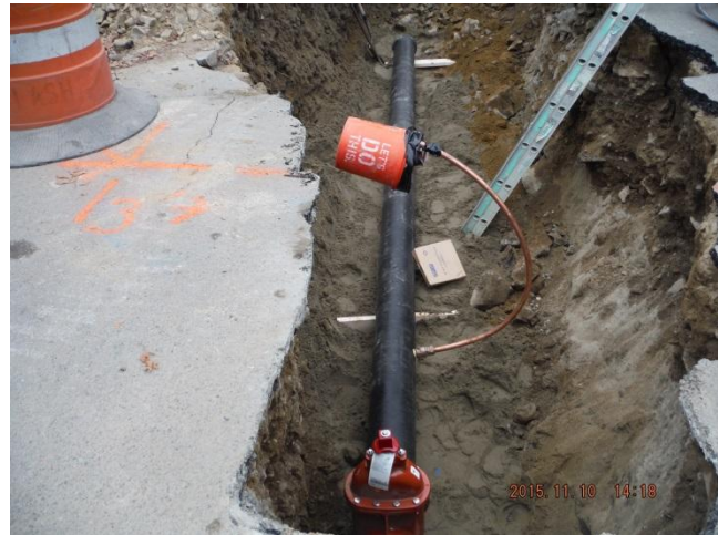
New Water Main with blow off installed for pressure and chlorination testing 11/10/15
