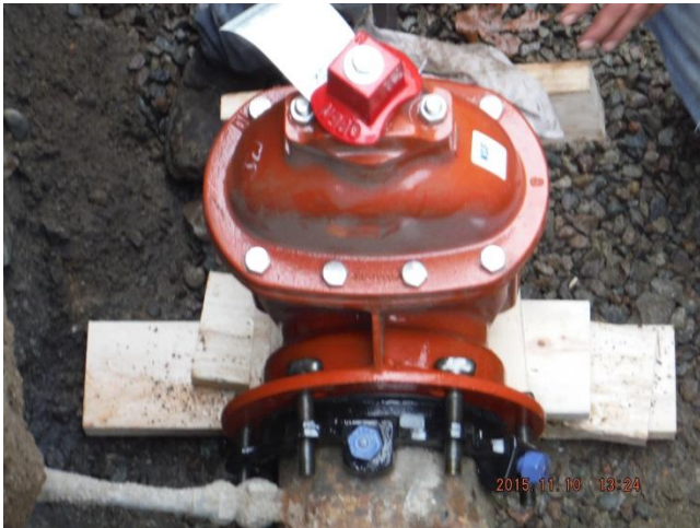
Connection to existing water main and Install shut of valve STA 0+28 Rockwood Lane. 11/10/15
