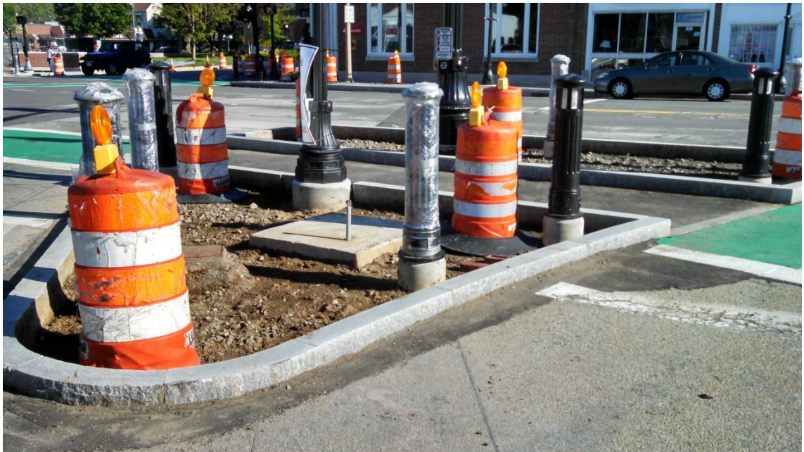
Dedham Ave. island prepped for concrete base installation for granite and brick pavers
