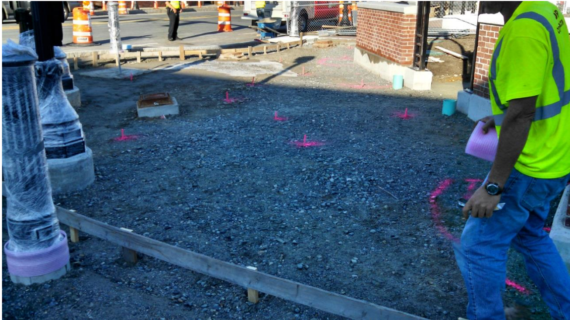
East side of the Common prepped for concrete walk and granite and brick paver base
