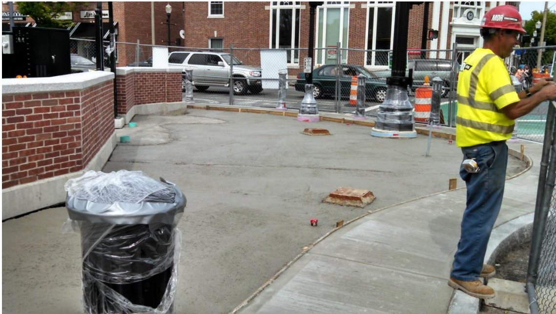
East side of Common after concrete sidewalk and base for pavers is placed
