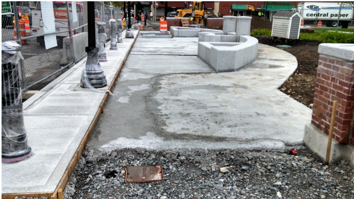
Concrete sidewalk and brick and granite paver base slab in front of Common looking west
