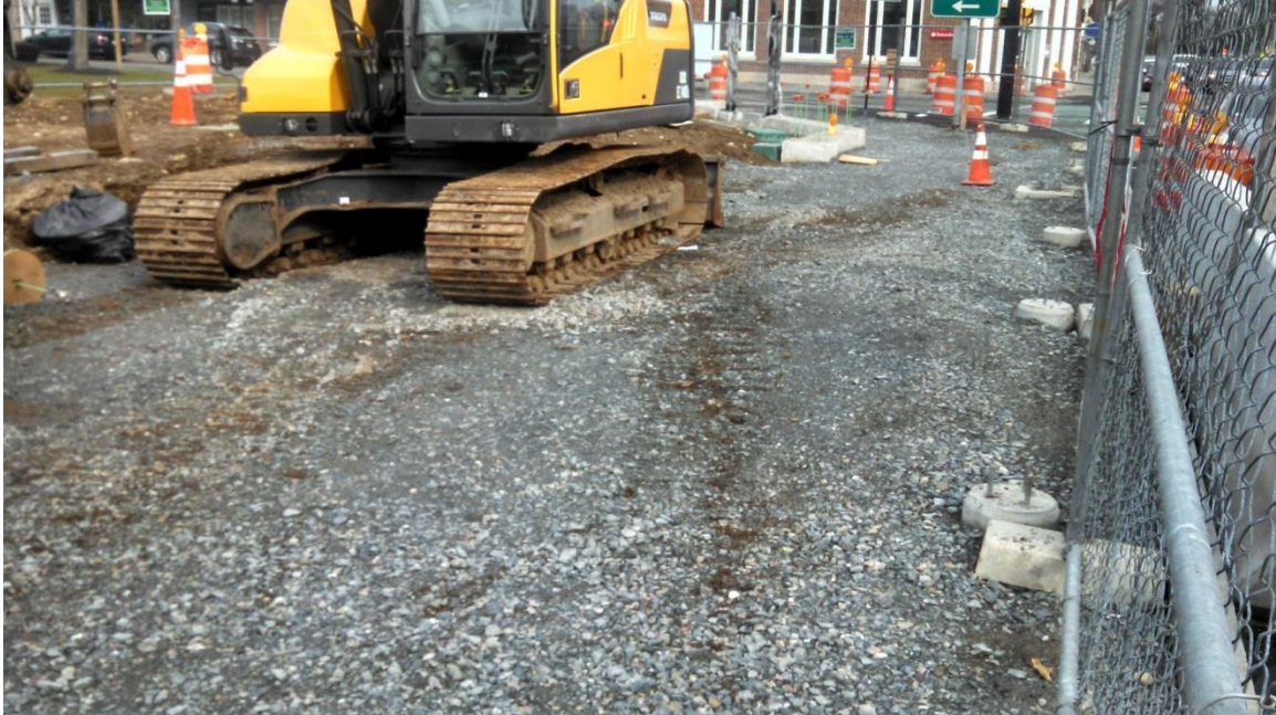
Gravel base installed for granite seat wall and brick paver installation in Common
