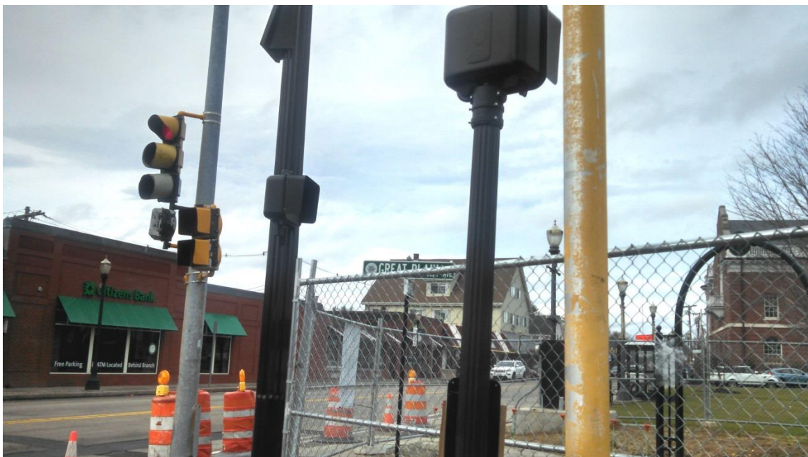
New mast arm posts and pedestrian signals installed at the northeast corner of Great Plain Ave. and Chapel St.
