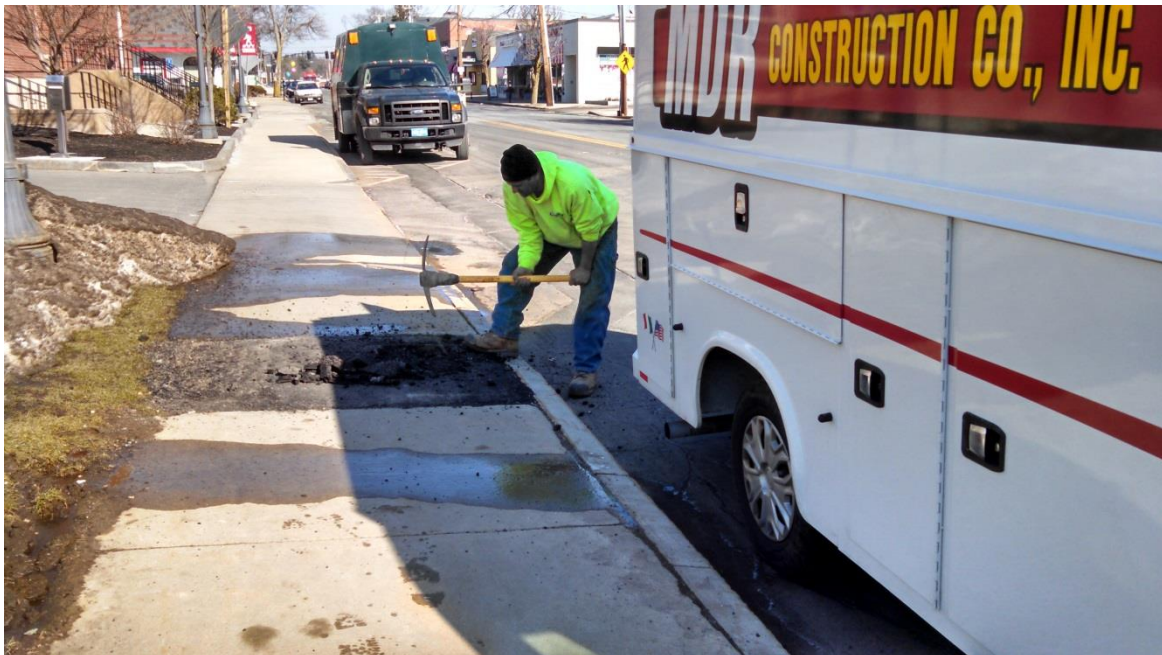
Chipping out and raising the conduit hand hole frame and cover to raise it to grade in Highland Ave.
