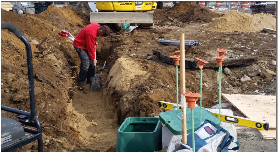
Installing conduit and hand holes for various electrical equipment in the Common
