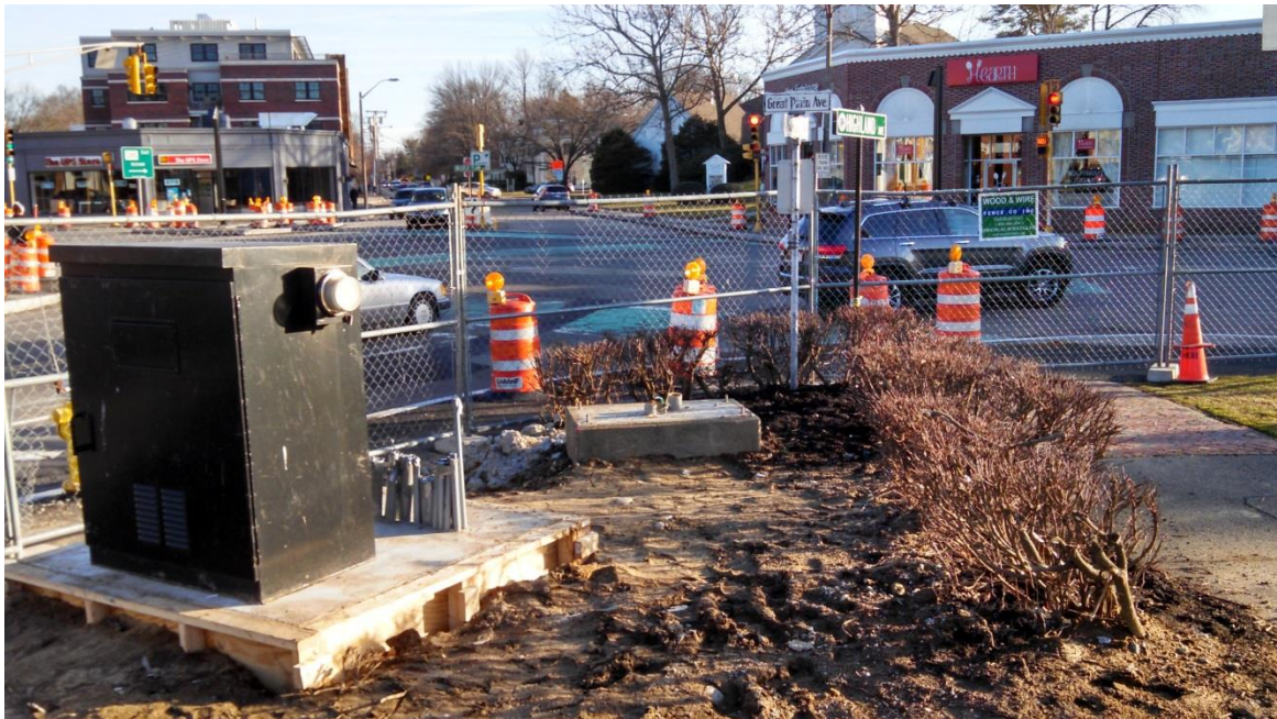
Existing traffic signal control cabinet temporarily moved on the Highland Ave side of the Common
