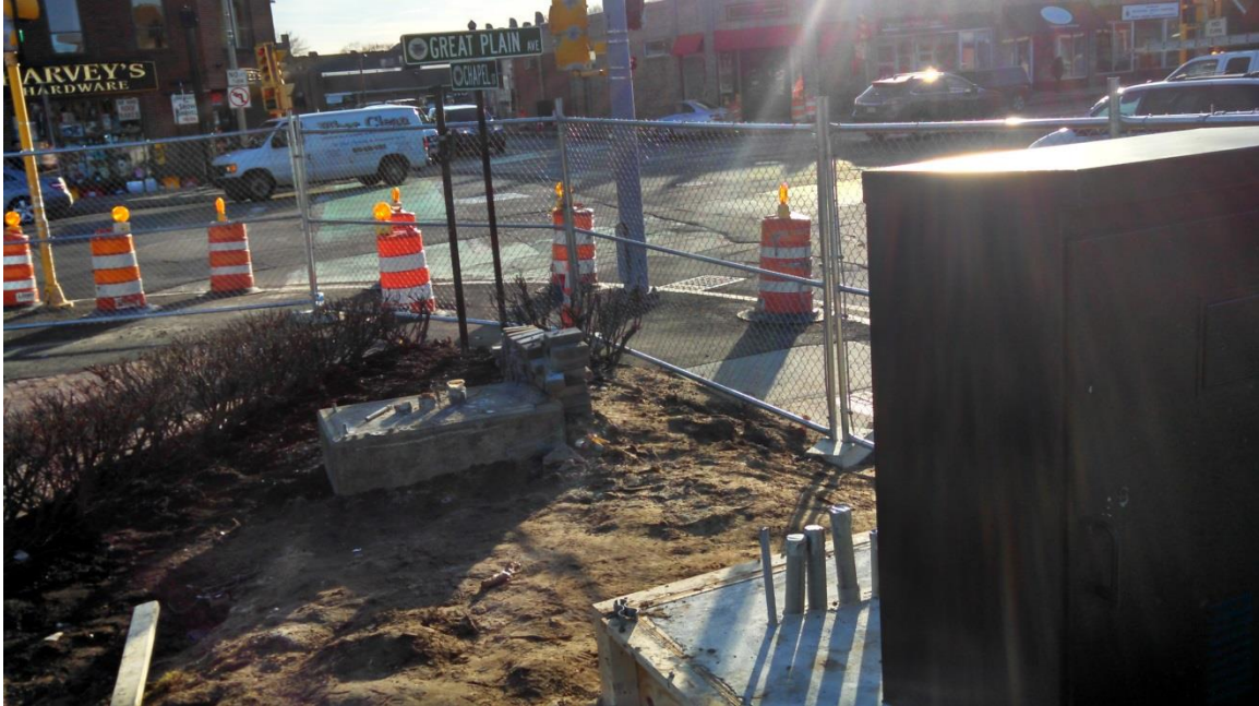
Existing traffic signal control cabinet temporarily moved on the Chapel St side of the Common
