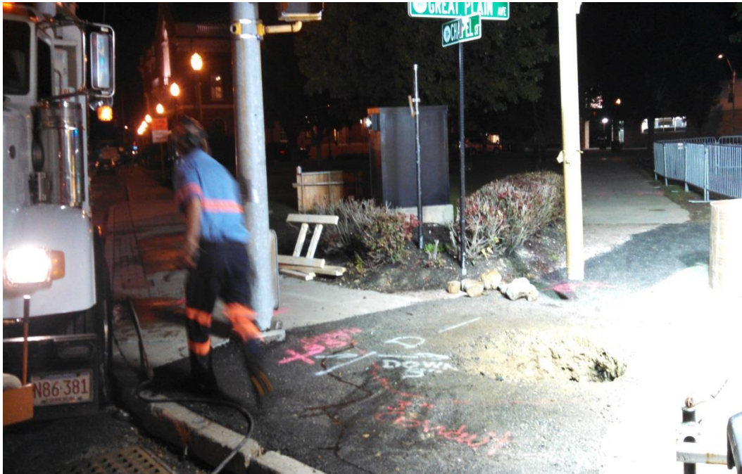
Excavating for mast arm and control cabinet foundations using a vector truck
