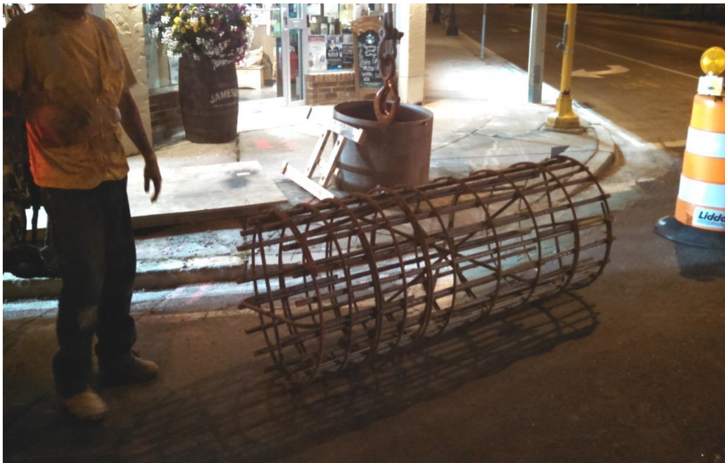
Preparing to install the reinforcing cage for the mast arm foundation on the corner of Great Plain Ave. and Chapel Street
