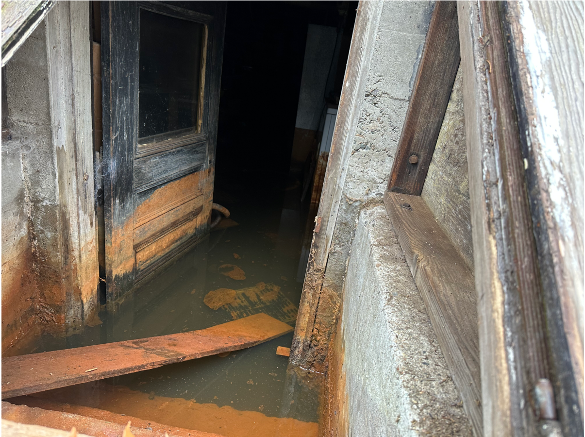
EXHIBIT C Photo of Flooding in House Basement
